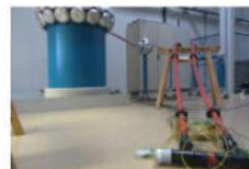
Figure 3: Ready for DC voltage measurement
